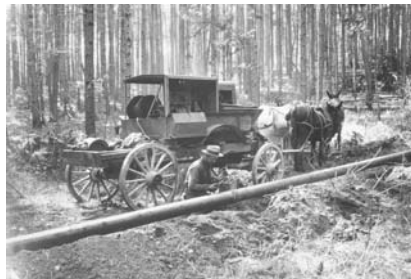
September 1927 – Lamkin Hodge Pipeline. Getting ready to lay the final bead on a bell and spigot joint for this 8-inch line which carries gas from Lamkin, Louisiana to Hodge, Louisiana. This was one of the first major pipelines to be arc welded, and Lincoln equipment was used exclusively for this project.
